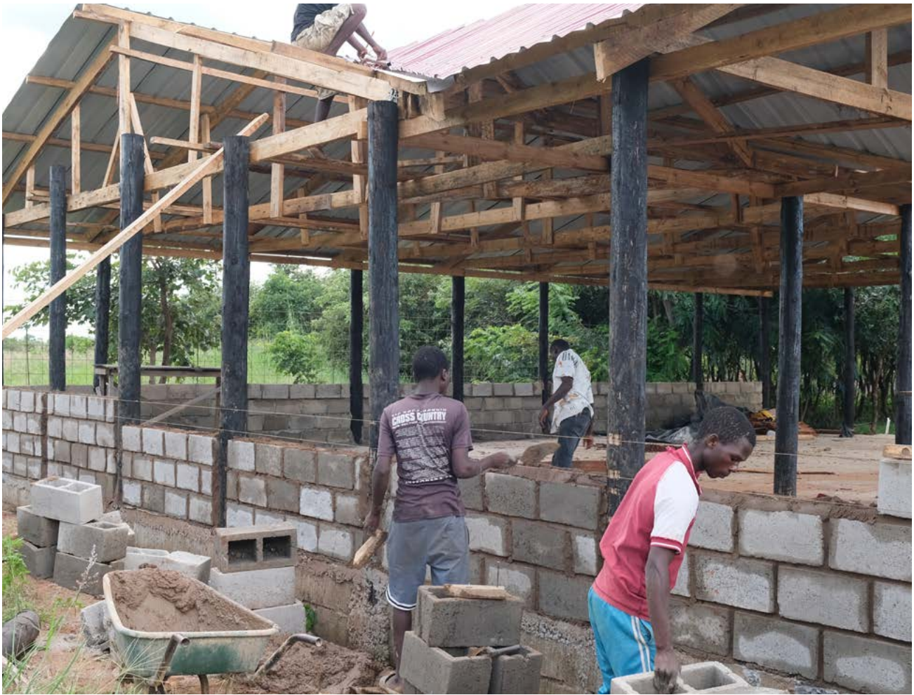
■ Construction crew building the workshop's outer walls and finishing the steel clad roof. Kuwala_2024.
