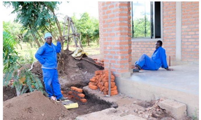
■ Water drainage around the St. Peter's Assembly Hall foundation helps with drainage in the rainy season which in 2022 resulted in extensive flooding in Malawi. This is one of the ways we prepare for extreme weather events. Kuwala_2022.
